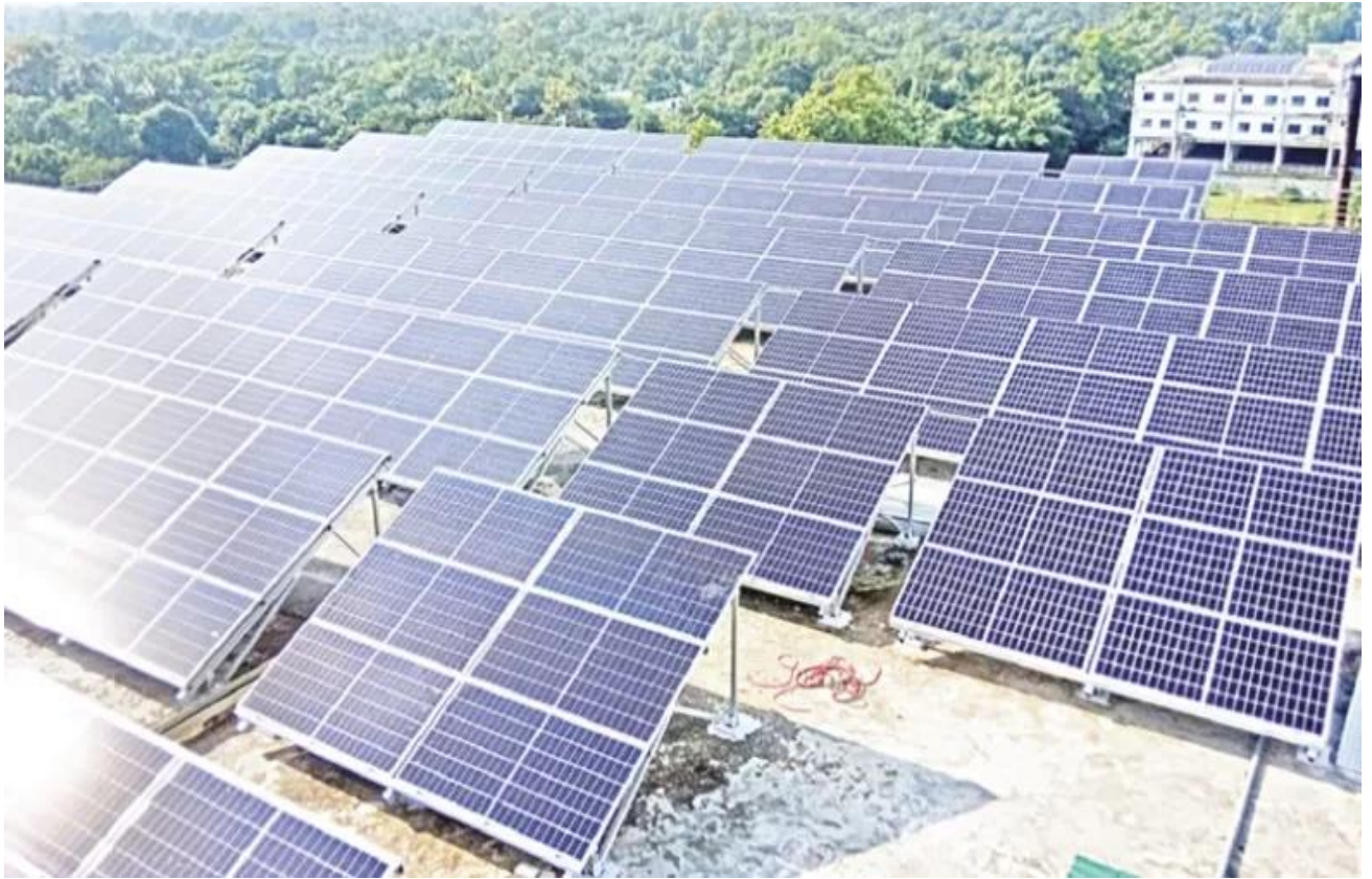
The picture shows solar panels installed on a rooftop – Collected Photo
